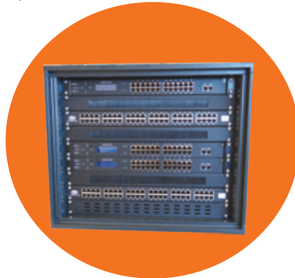
INSTRUMENT ROOM 9U PHONTECH SYSTEM CABINET
