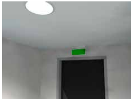
Emergency escape signs
